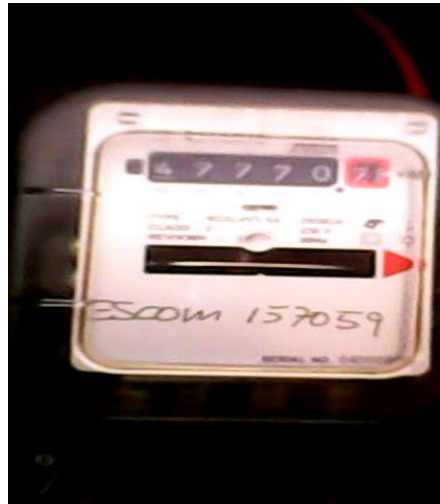
Figure 11.45 Electricity board's meter
